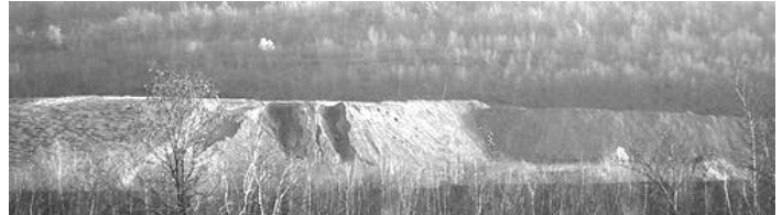
Deep erosion gullies from erosion of "cement-like" waste coal ash dump in Schuylkill County, PA
